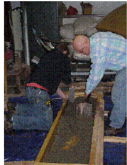
The forms were filled, leveled, numbers placed in the concrete and left to cure for a week.
